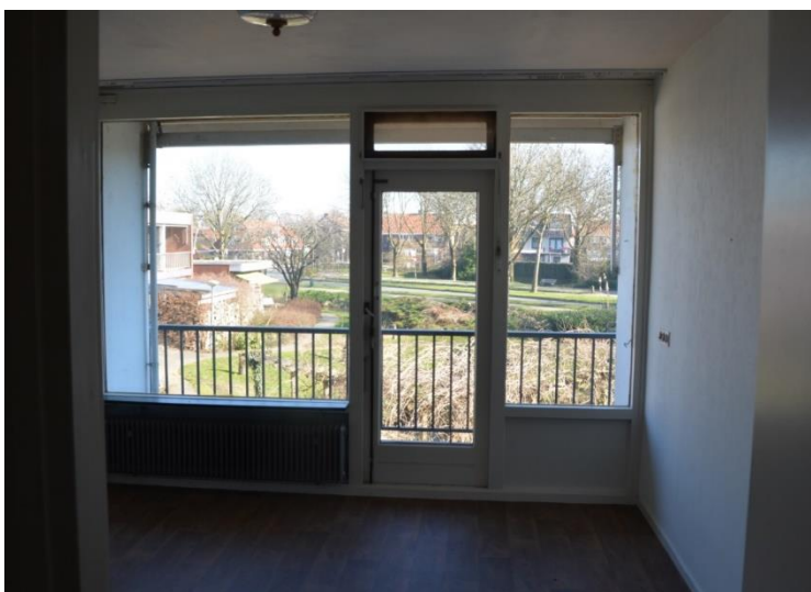
Figure 1.4 Picture of one of the fire rooms
