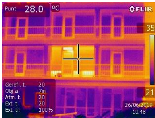
Figure 6.5 Thermal imaging camera (TIC) images of test 4 of variant 1 (door closed)
