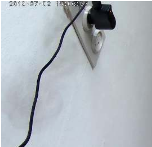
Figure 3.32 Smoke propagation via a wall socket with a central antenna connection in residence 2.19 during test 13 of variant 5
