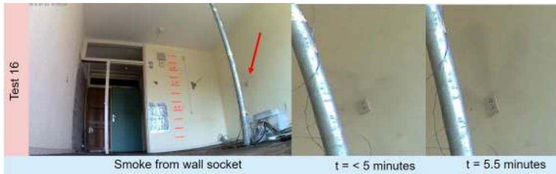
Figure 3.8 Smoke from a wall socket in the wall of residence 1.20 during test 16 of variant 1
